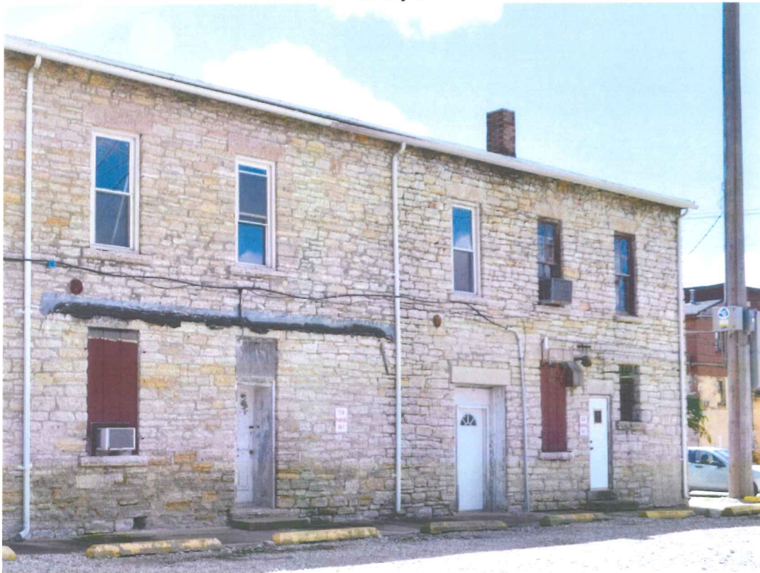
Detail of windows on north façade; note vinyl replacement windows to the left/east and original windows to the right/west. The door opening to the east appears not original.
