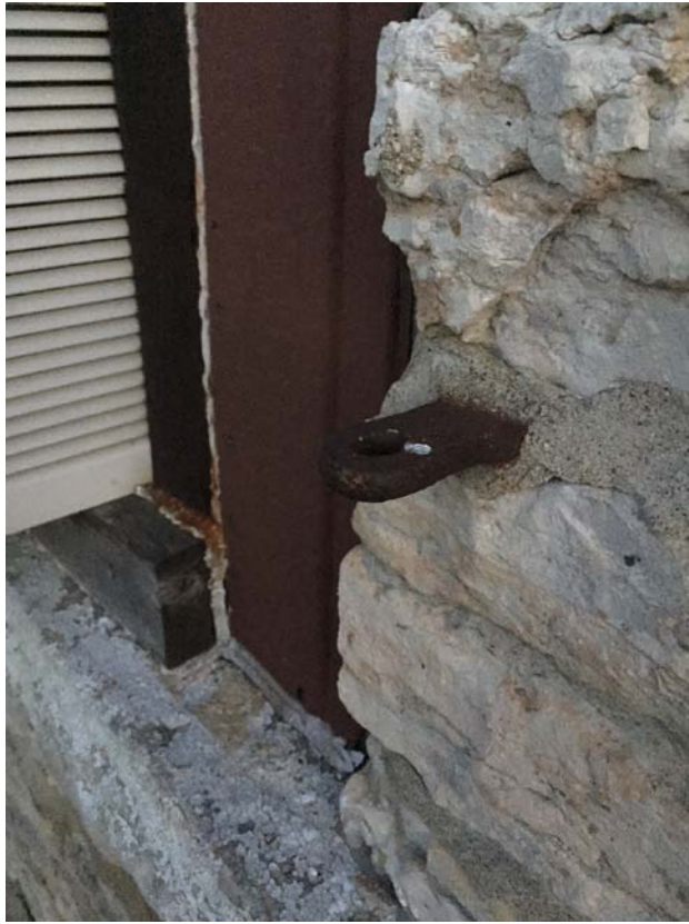
Four metal “loops” (two on each side, high and low) are present next to the window openings on the south façade, rear façade window and door, and north façade lower windows.
