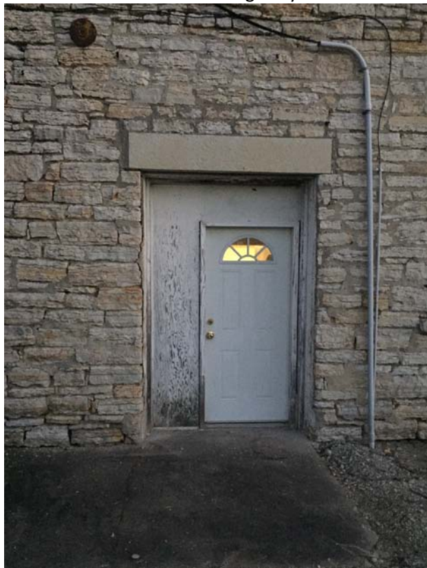
On the north façade, one door opening appears to have been modified from its original configuration.
