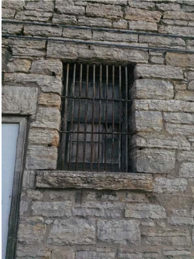
Metal bars still exist on some of the exterior window openings.
