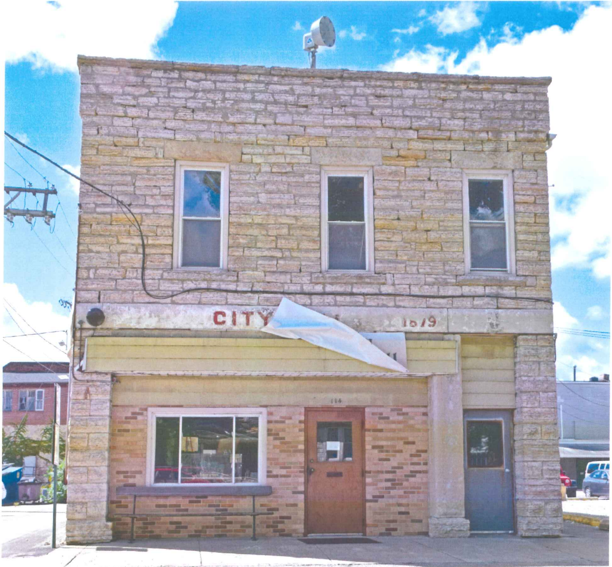
East/Main Street facing façade; alterations include closing in the large garage door opening, window replacement on the second story, and door/transom replacement to the right/north.
